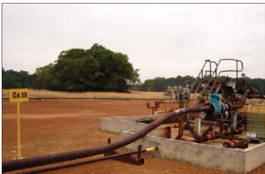
On each gas-lift well, the monitoring system measures tubinghead pressure, casinghead pressure, tubing temperature, differential pressure (gas-lift flow line), and annulus pressure (Fig. 2).
