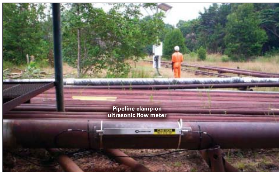
One of the new subsystems installed was a pipeline ultrasonic flowmeter (Fig. 6).
